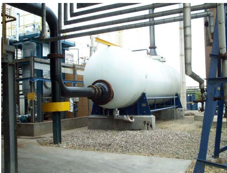
Figure 6. New quench tank
