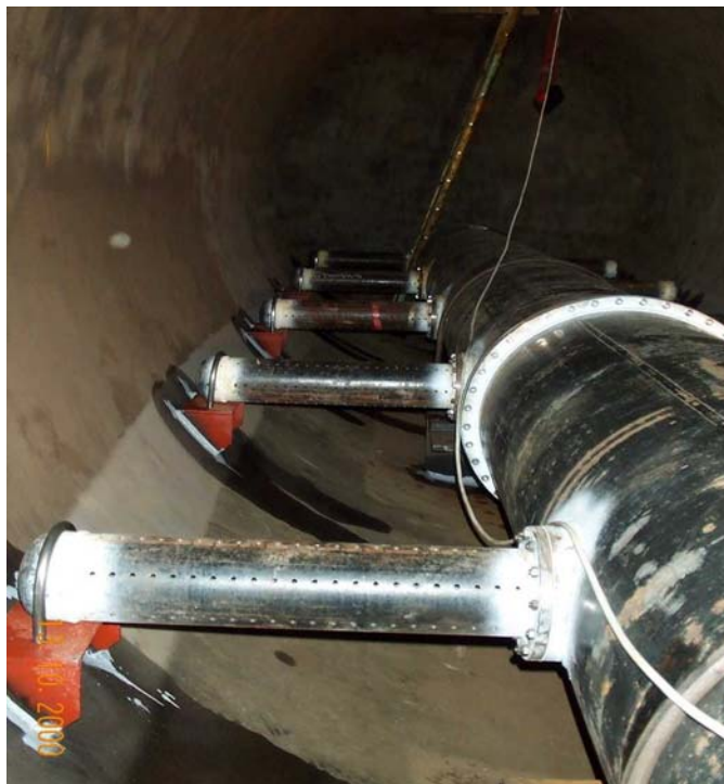
Figure 5. Sparger inside new quench tank
