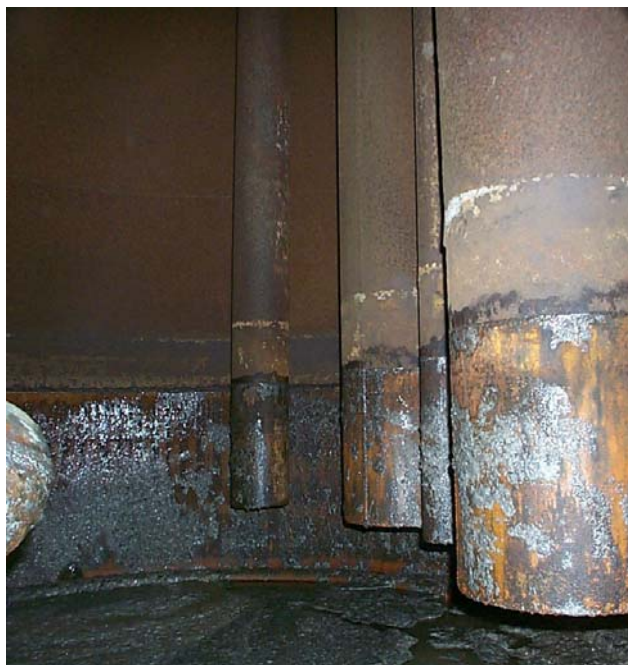
Figure 2. Inside of V7 after incident
