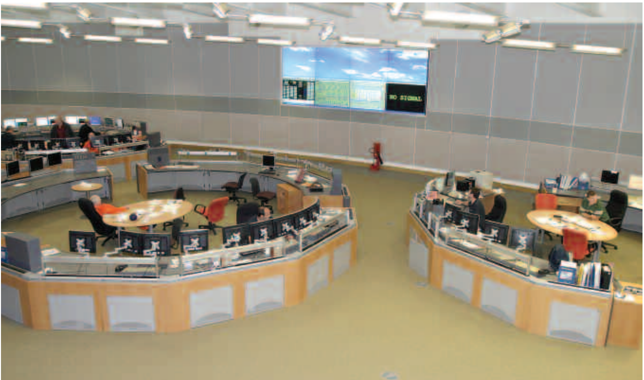
Figure 9 A modern process control room
