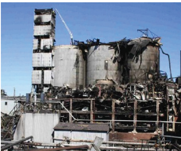
Figure 3: The damage to the south packing building and the penthouse
