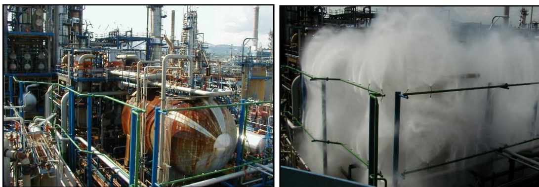
Figure 6. Water Curtain Mitigation Prior to and during Activation
