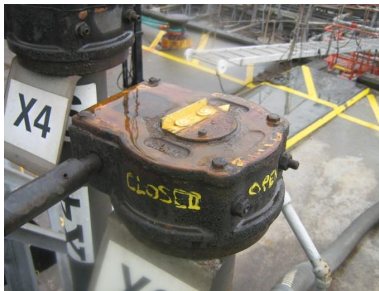
Figure 5 Picture of the Jetty Valve
