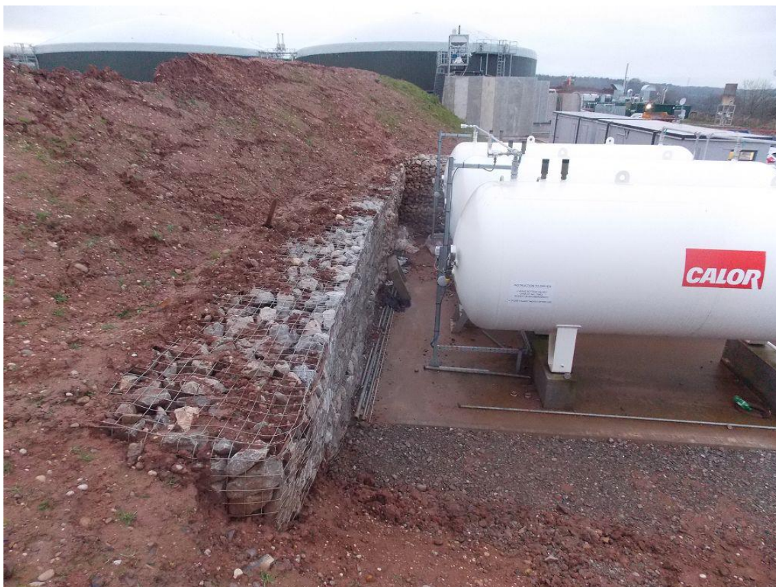
Figure 8: Bund collapse towards Propane Storage.
