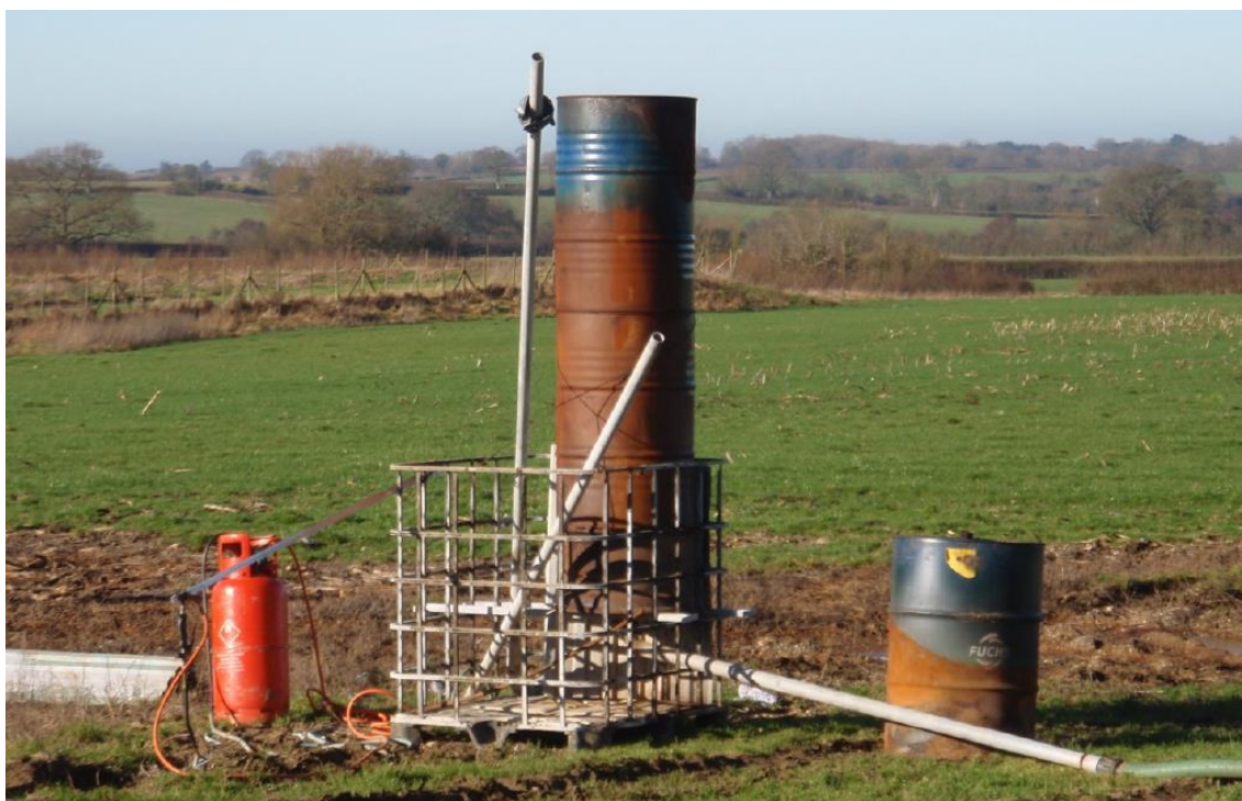
Figure 10: Unconventional Flare used on Agricultural AD plant. Source: (Environment Agency, 2018)
