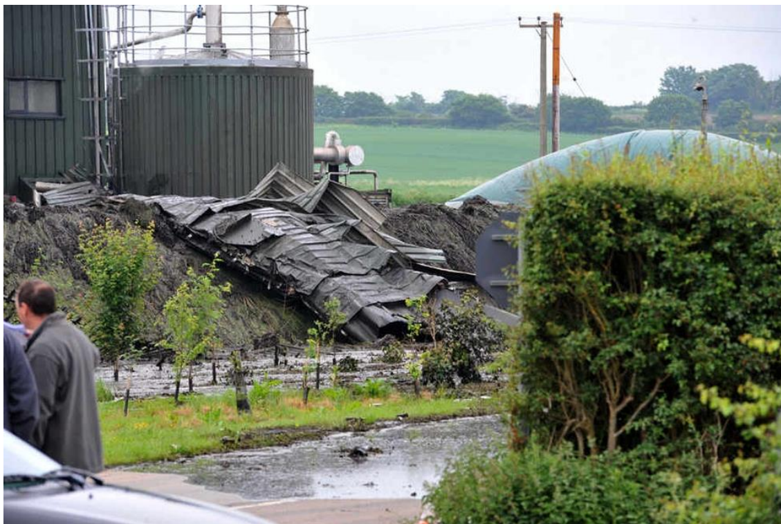
Figure 7: Tank Collapse and subsequent Loss of Containment. Source: (Environment Agency, 2018)
