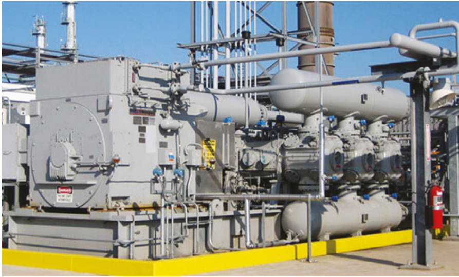
Figure 3: Ariel model JGU/6 hydrogen compressor – Air Products & Chemicals.
