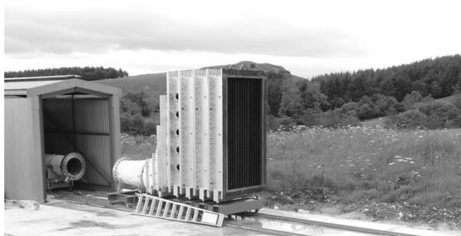
Figure 3. Image of HRSG under construction, showing open exit from circular duct. The first 3 sections of the HRSG and the 3 sections of the heat exchanger are shown.
