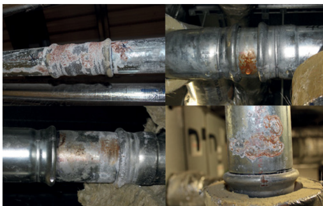
Figure 4: Examples of lightly corroded galvanised TWCS pipework are shown below
