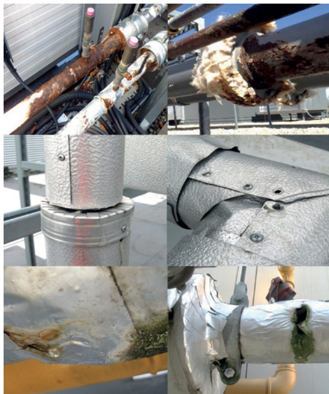
Figure 3: Examples of rooftop pipework CUI problems and poor insulation installations are shown below
