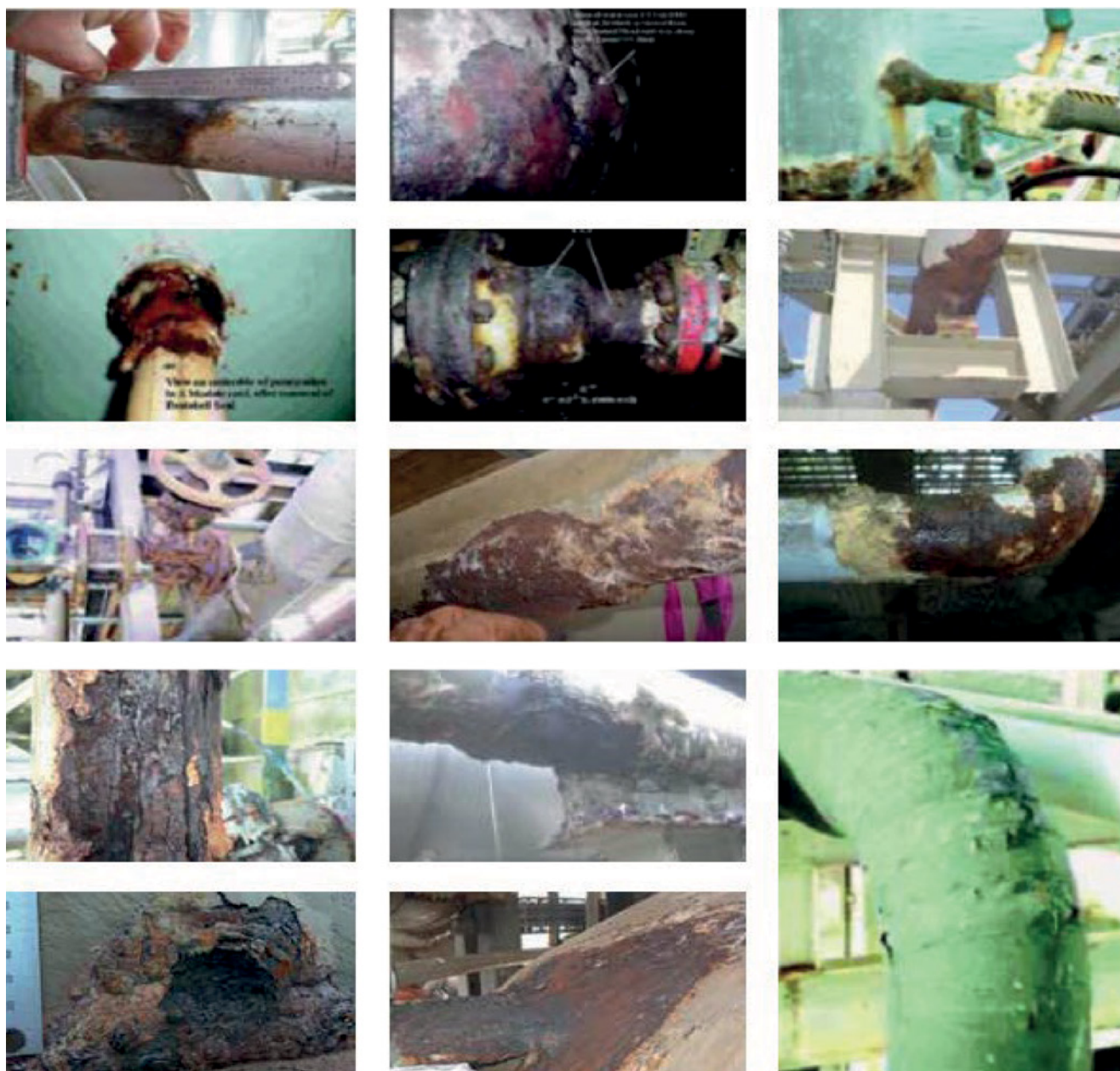
Figure 1: Images of CUI (Reproduced with kind permission from the Energy Institute from their Guidance on Corrosion Management 1 )
