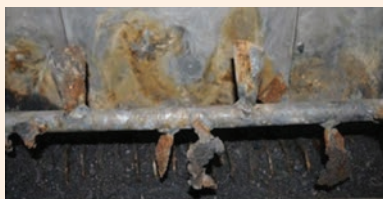
Press Blade Damage
