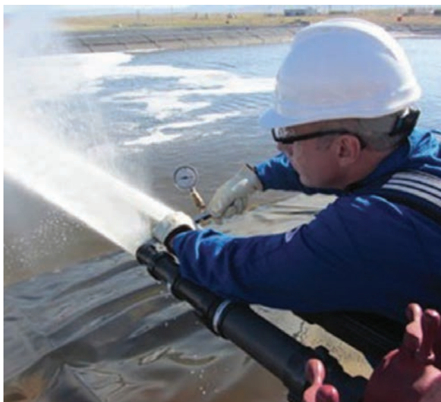
Figure 2 – Firewater flow measurement
