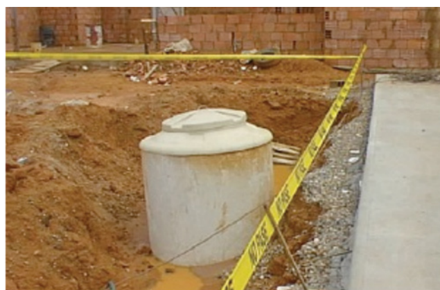
Figure 3: Underground tank with entry forbidden
