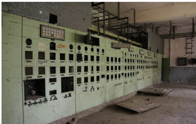
Control Room Feb 2014 (Credit BMA)
