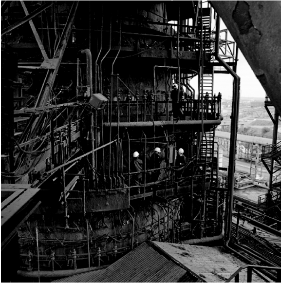
Figure 5: External view of the furnace cooling system
