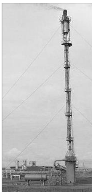
Figure 1. A guy supported onshore elevated flare stack showing from L to R – flare knock out drum, integral seal drum, flare stack and flare tip with a molecular seal (large diameter component) visible just below the flare tip.
