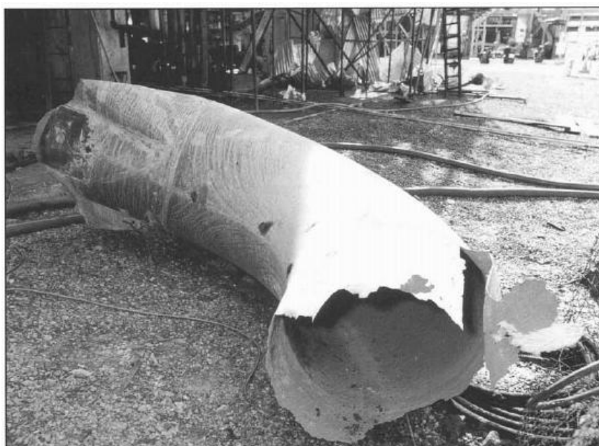
Figure 3. Corroded elbow on a 30 inch diameter flare header which failed due to the impact of liquid hammer following a flare knock-out drum overflow, Pembroke Refinery & Cracking Complex, 1994.
