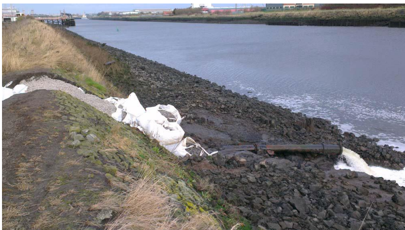
Figure 2. Inter Terminals, Riverside Terminal. Damaged flood defence embankment showing the temporary repair.
