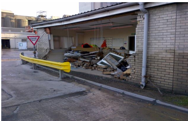
Figure 11. CEMEX – wall collapsed due to pressure of floodwater.
