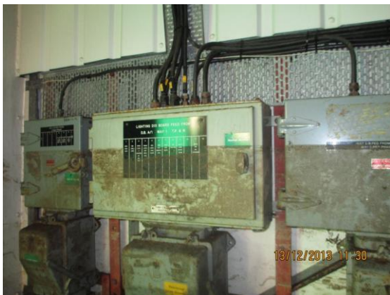
Figure 6. SABIC - flood damage to electrical equipment.
