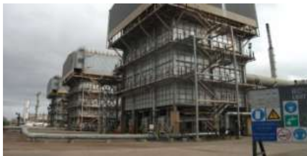
Photograph 1 – Primary Reformer Furnace
