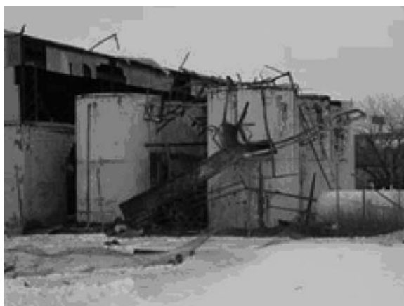
Figure 8. ASCO: damage and debris around the decant water tanks
