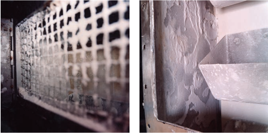
Figures 5 & 6. Photographs taken looking into the hatch on the Import/Export Elevator showing heavy build up of sugar on walls and up-leg of Silo Feed Elevator through hatch at Level 2.5 showing residual sugar fines on casing wall and bucket and less evidence of caramelisation
