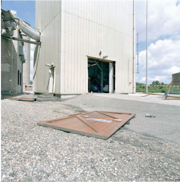
Figure 10. Building housing Airmaster filter. Note damaged ductwork at 3-way junction
