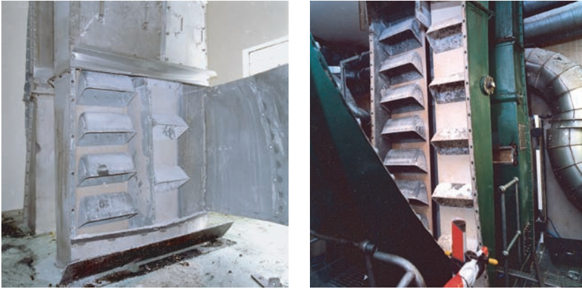
Figures 8 & 9. Damage to Production/Bulk Export Elevator on level 2 to Production/Bulk Export Elevator just above ground level
